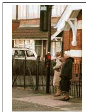
PDU at the back of a narrow footway
