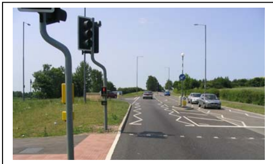
PDU's incorrectly installed on the leaving side
